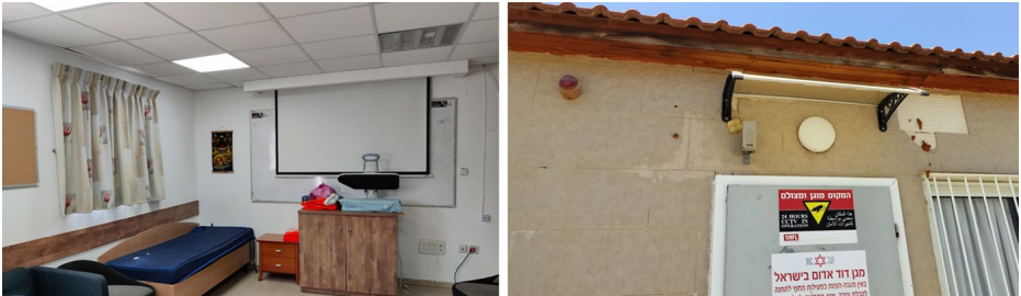
(Left) The station's only changing room, (Right) Damaged exterior tiles
