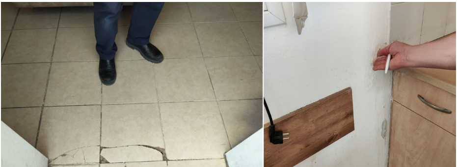
(Left) Broken floor tiles, (Right) Damp damage to interior walls
